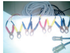
Two Set of 10 m Long Three Phase Cable
